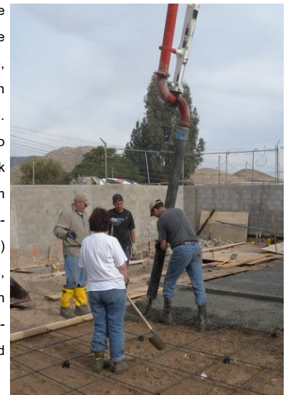
Scott Emley working hard at pouring the cement (that looks heavy!!). Jon Funk, Sue Rice, and a local worker waiting to flatten it even. It took a lot of effort to make this happen!
